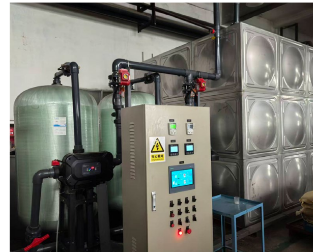
Dongying Factory Water Softening Ion Exchange System
